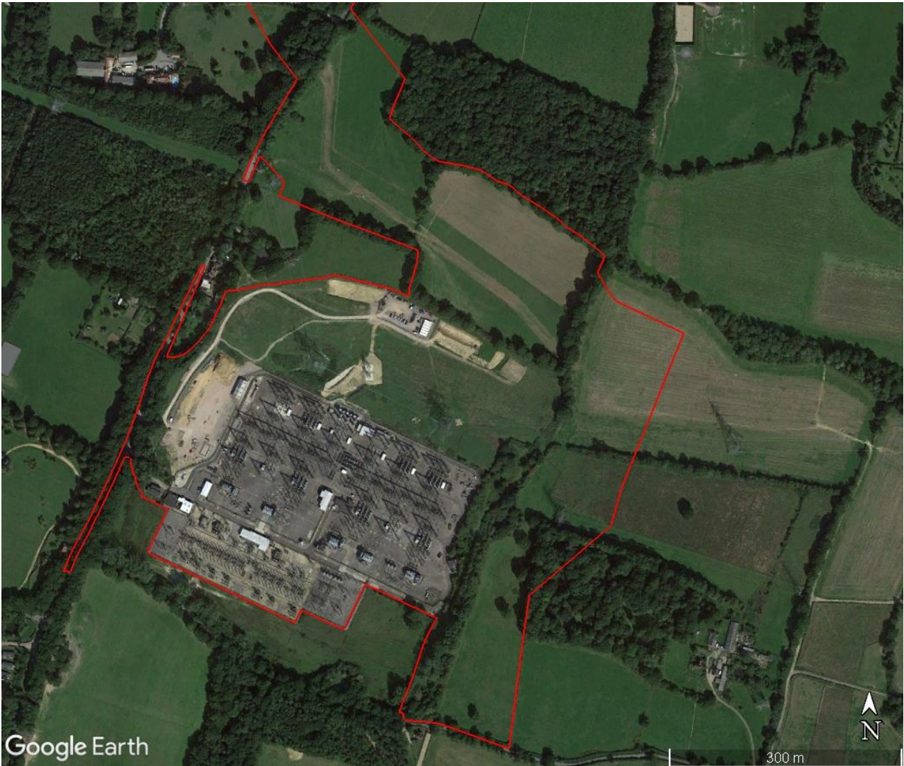
Plate 7 2015 satellite image showing works at existing National Grid Bolney substation (Google Earth)
